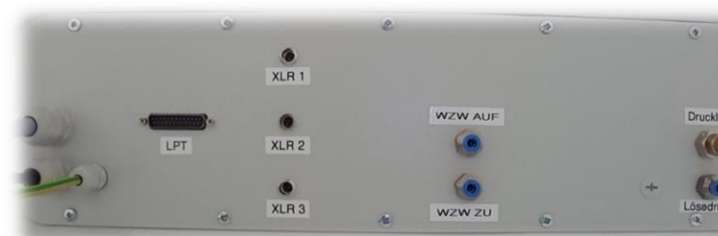
Switch Cabinet ATC-8022-42
