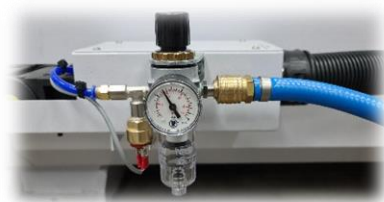
Fig. 10.5: Pressure control valve with pressure monitor
