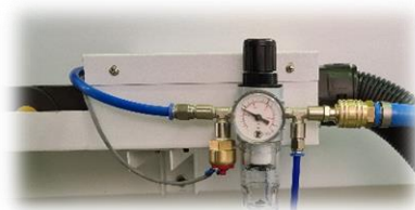
Fig. 8.4: Pressure control valve for cylinders
