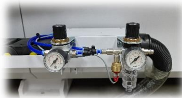
Fig. 10.6: Two pressure control valves with pressure monitor
